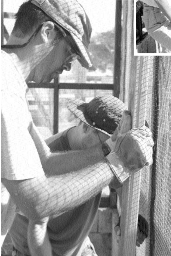
Reconstruction of the cage system. Here Joel Friesch fits a new stud divider to split each large cage into two sections. Alberto Alvarez assists in background. Photograph by John Binns.
