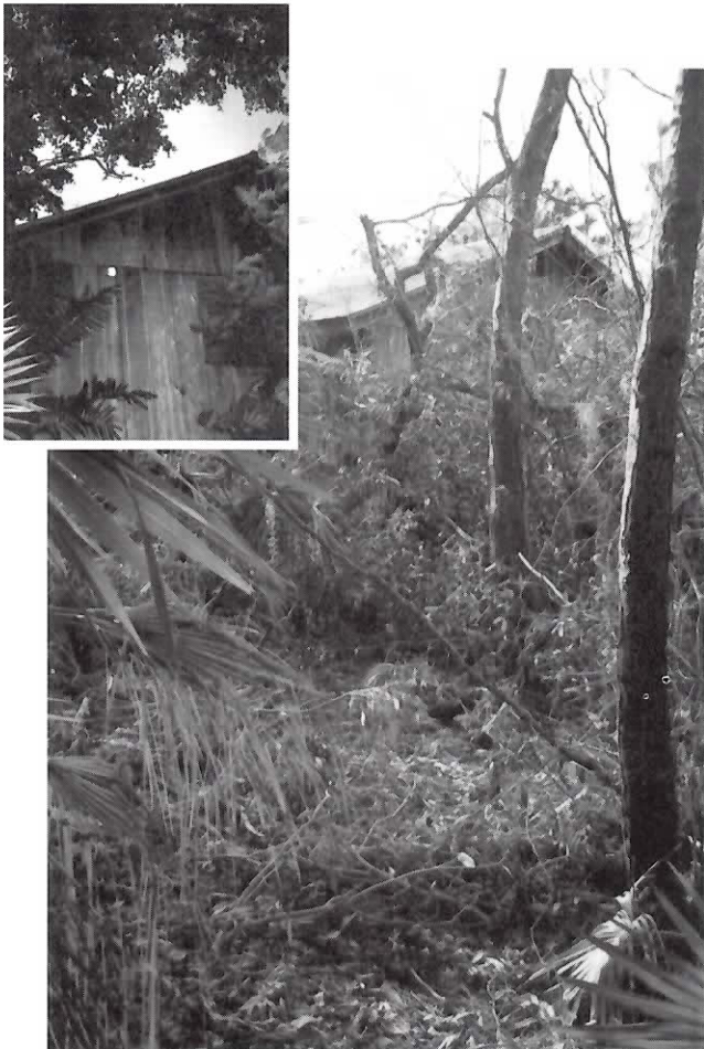
BEFORE (inset): Large black olive, Bucida buceras , towers over the house at the start of the storm.
