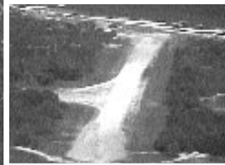
Inset: Construction of a runway for a new international airport and the accompanying development for
