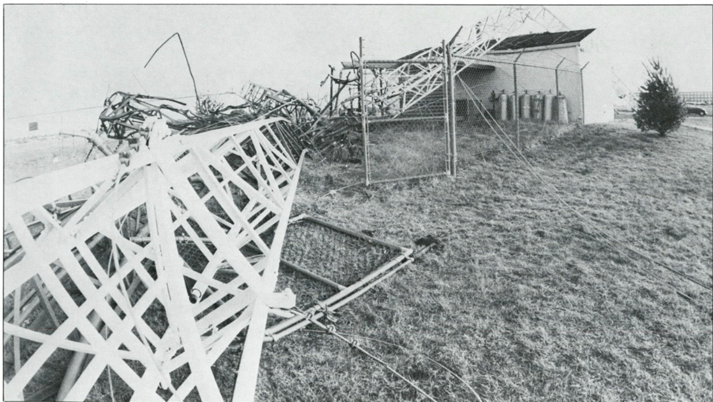
The collapsed tower left a pile of debris that cost $5,000 to remove.
