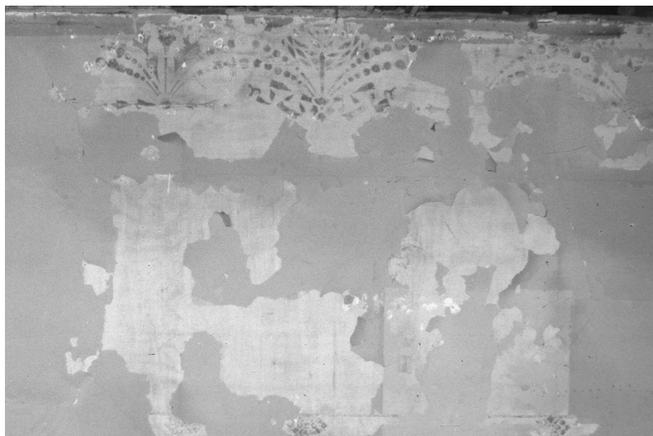
Figure 10. Interior view of Constitution Hall, showing remnants of wallpaper and paint.
