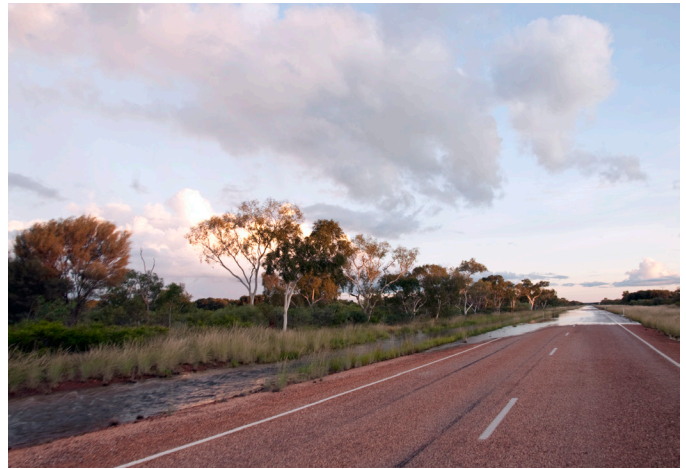
A flooded section of the Stuart Highway. Record flooding in Queensland in 2010–2011 made international headlines, and parts of the Northern Territory also received record rainfall, causing modest flooding like this. Photograph by Crystal Kelehear.
